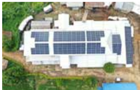
Factory rooftop solar - Bearwell Estate
